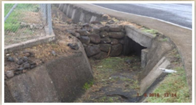
Figure 4: designed drainage and mount of boulders used to divert storm water into an underground channel.
