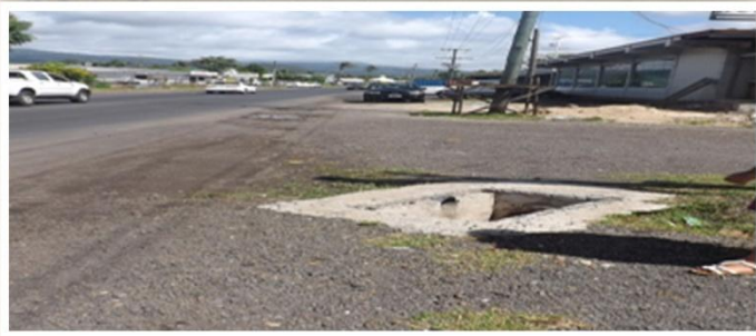
Figure 1: missing sump cover in front of Fugalei Tyre Centre
