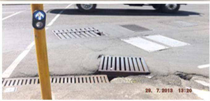
Figure 2: damaged sump cover located right along pedestrian crossing
